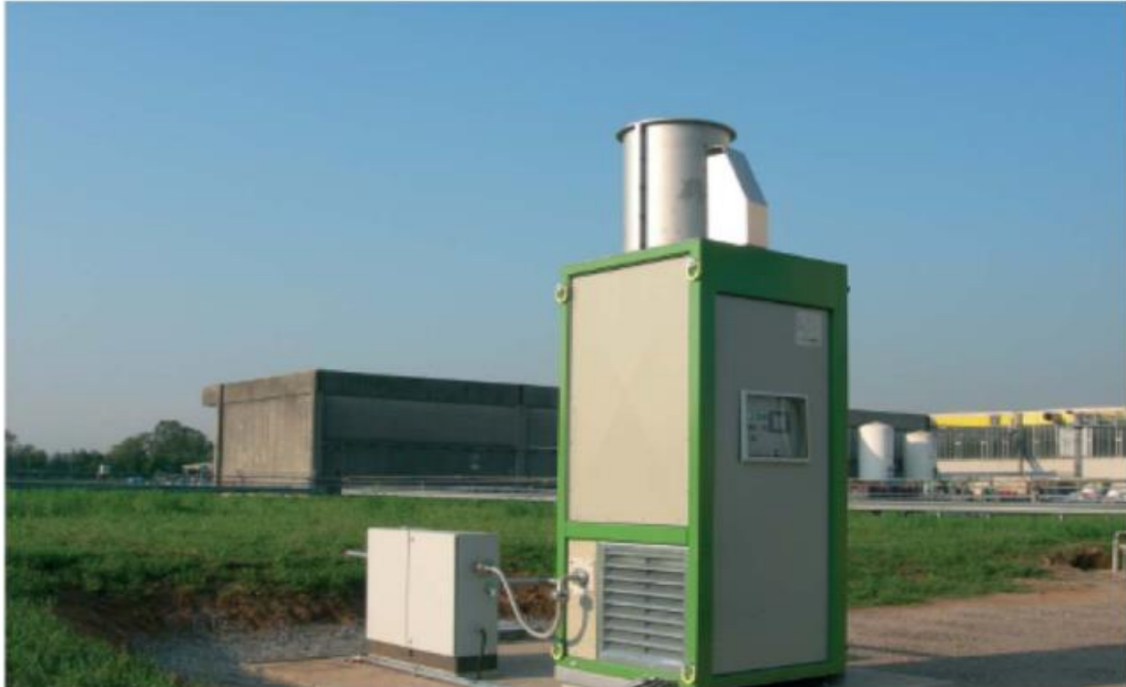
Photo of a CEB® 100 unit at a landfill
